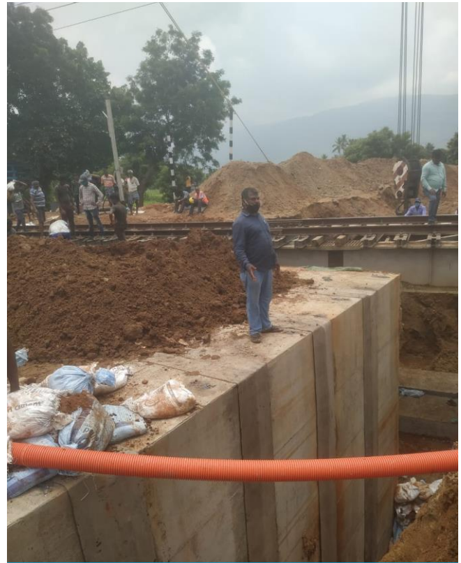
Side view of installation
