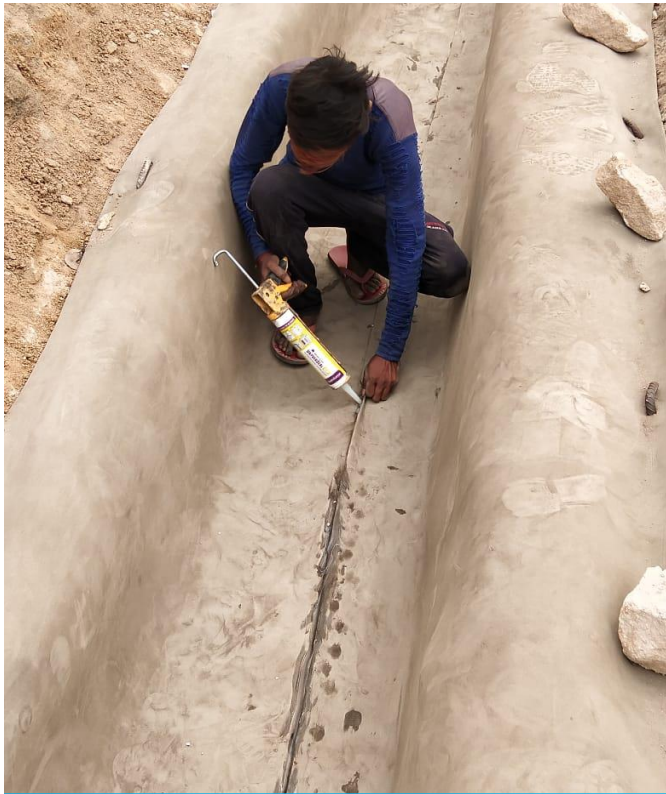
Existing choked nallah
