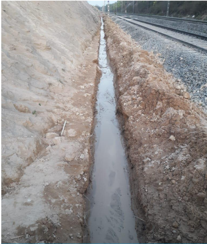
Existing choked nallah
