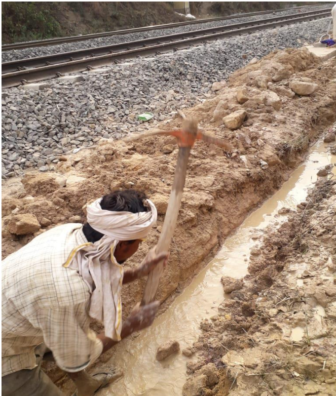
Existing choked nallah
