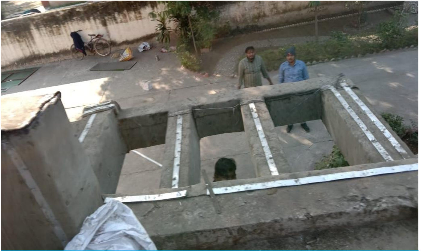
Top View of Completed Installation
