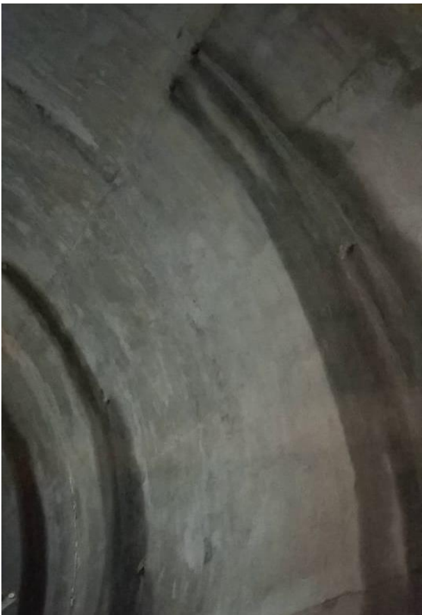
Leakages from top & side walls
