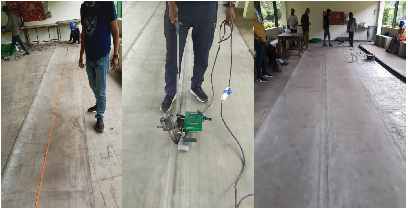
Cutting of CC5 as per measurement in length & thermal welding in width direction to widen it to 1.9m
