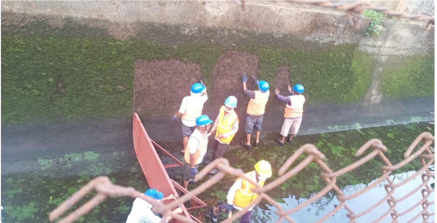
Cleaning of damaged surface of duct line from algae, moss, dust, undulations & moisture
