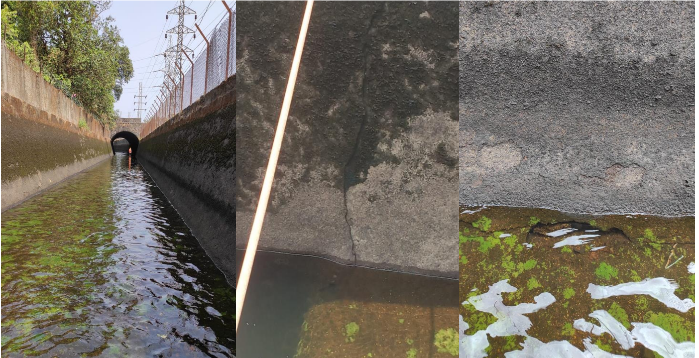
Photos Pain point of duct line showing cracked & eroded concrete lining
